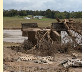
Destroyed bridge to Briar Thicket Baptist Church in Cocke County.
